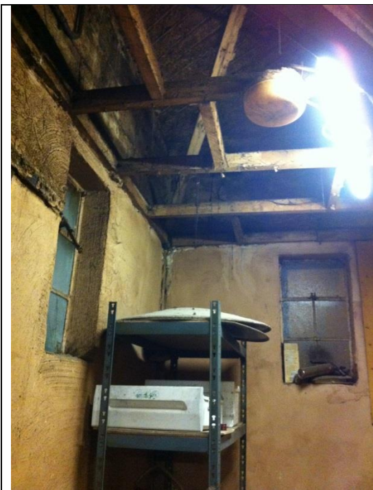
05 Rear store room in disrepair
