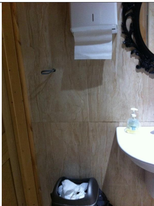
12 Exposed electrical cable next to wash hand basin in ladies WC
